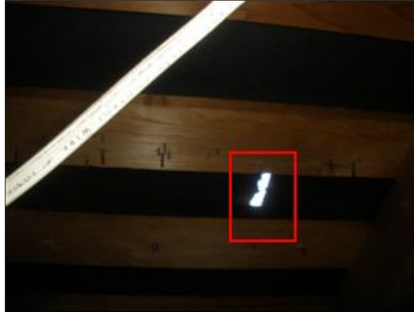
Item 1 - Picture 1 Roof hole above living room)
