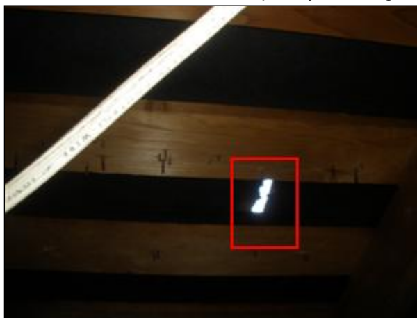
1.0 Picture 1 Roof hole above living room)
