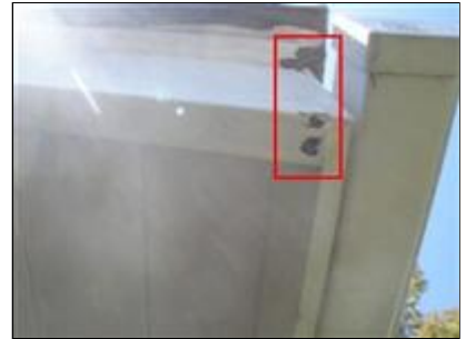
Item 5 - Picture 3 (Front left barge rafter and eave board)
