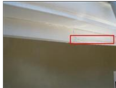
Item 5 - Picture 5 (Right front fascia board)
